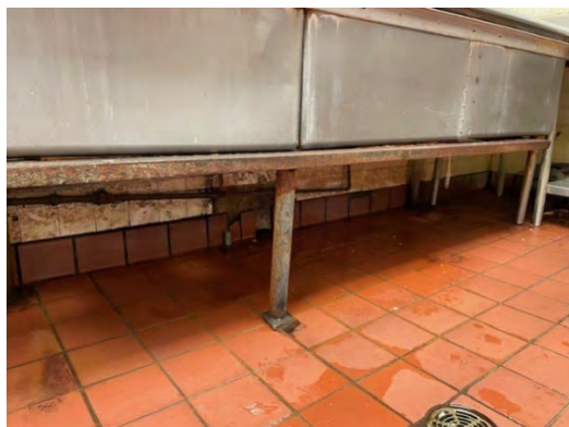
Rusted Kitchen Equipment
