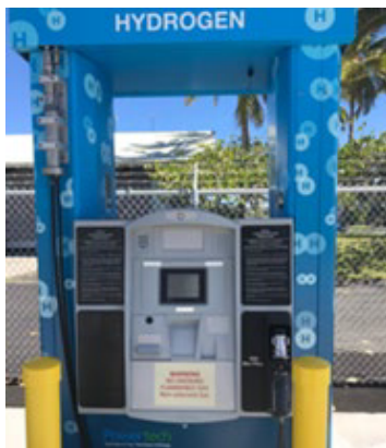
Figure 6. Hydrogen station dispenser.
