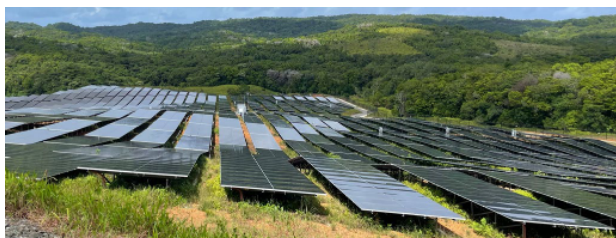
Figure 1. PV arrays at Palau's SPEC PV+BESS plant.
