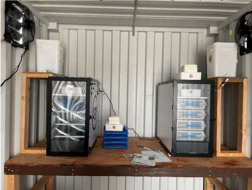
Photo 3. Cabinet incubator and hatcher in the EH Wildlife programs hatching/brooding facility. Electrical and ventilation were installed during FY24 using WLRF.
