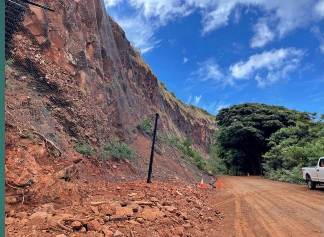
Ko Road Central Mauka Rockfall Mitigation, Kauai— Attenuator drapery netting system installed in Fall 2023
