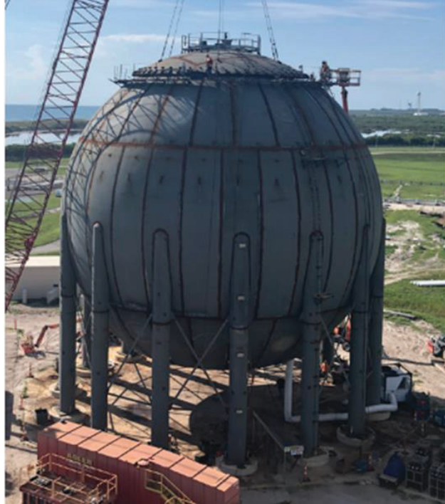
Figure 7.4. NASA 330 metric ton large-scale liquid hydrogen storage tank 16 .
