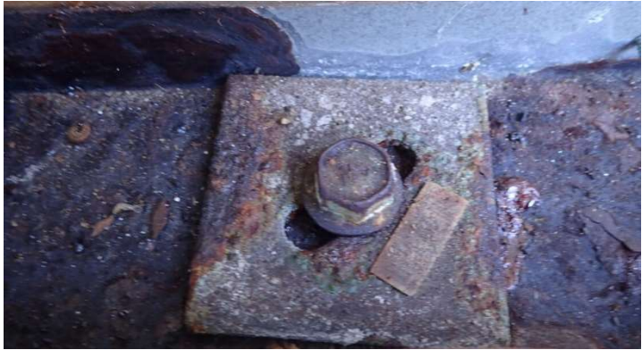
Corroding sill track
