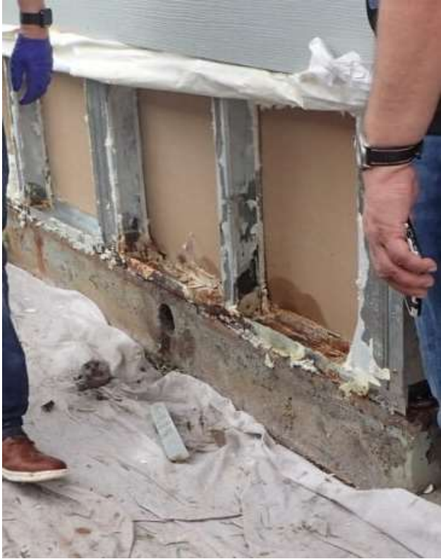
Rusted sill track and anchor screw
