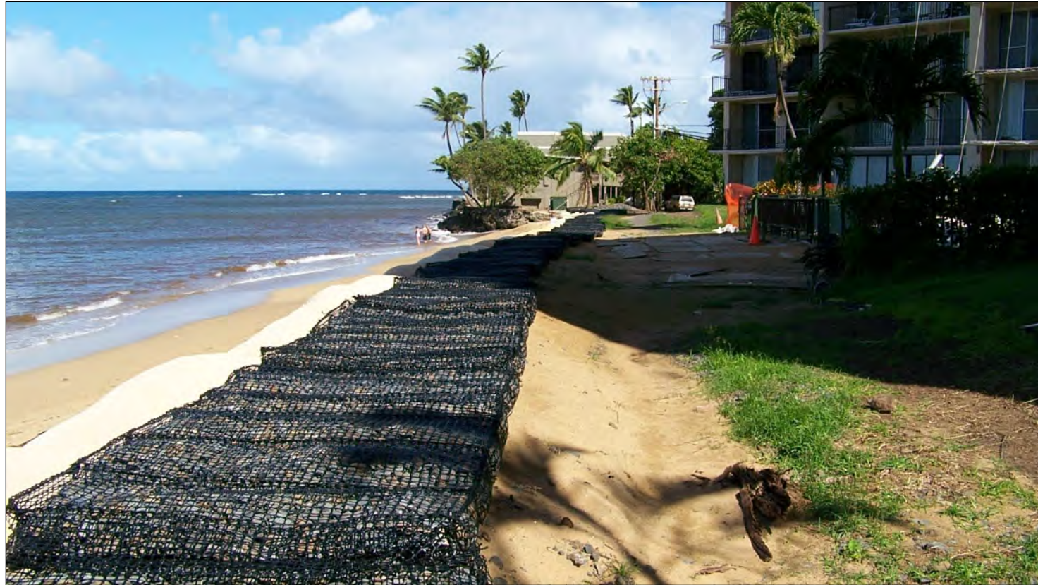
Photo: Tensar geotextile mattress filled with hard, angular rocks to capture sand particles.
