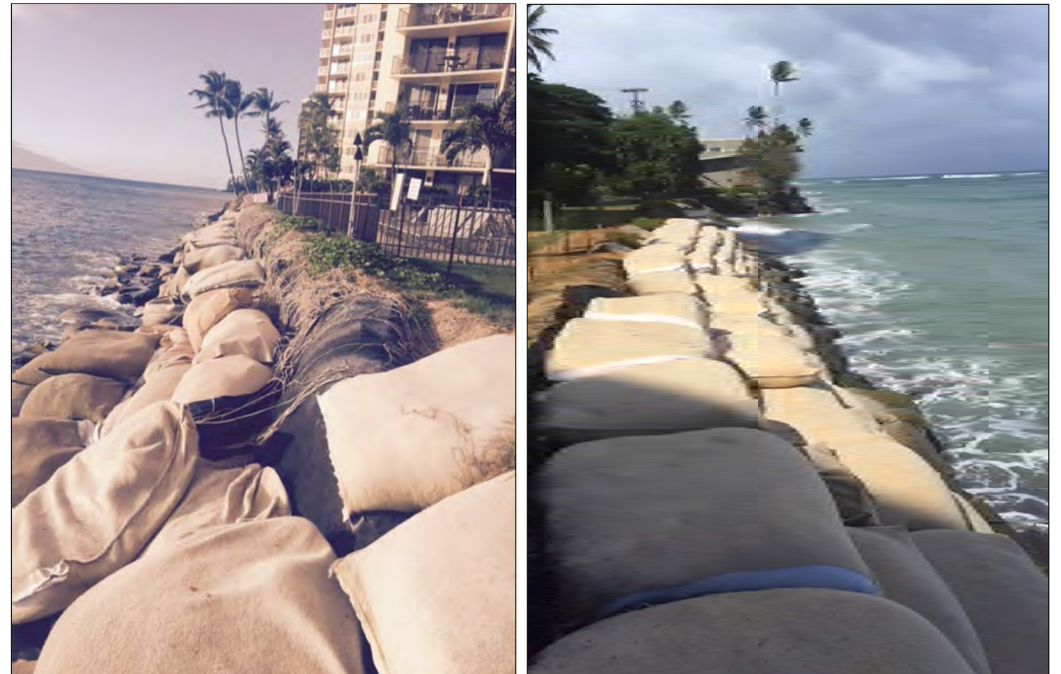
Photos: Geotextile bags may shift due to storm surge and typically require maintenance over time as these before and after photos illustrate, West Maui.
