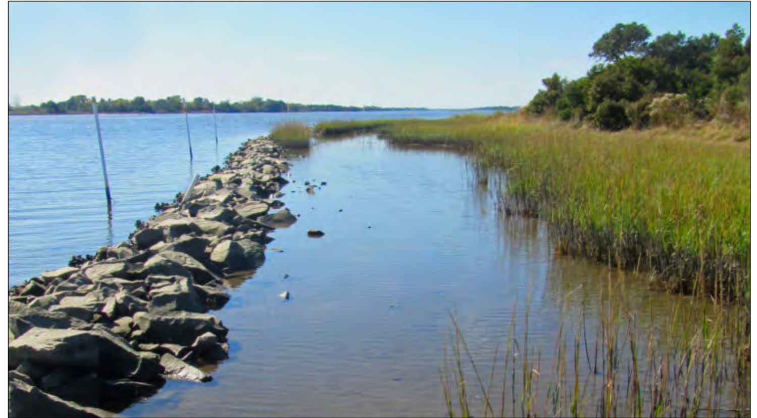
Photo: Breakwater sill and marsh vegetation at Morris Landing, Holly Ridge, NC. Photo: Carter Smith. Source: https://ncseagrant.ncsu.edu/currents/2018/11/living-shorelines-can-enhance-saltmarsh-resilience-to-hurricanes/
