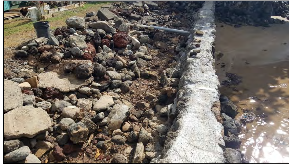
Photo: This wall's effectiveness could be improved with more weep holes distributed behind the wall and more porous aggregate as fill.
