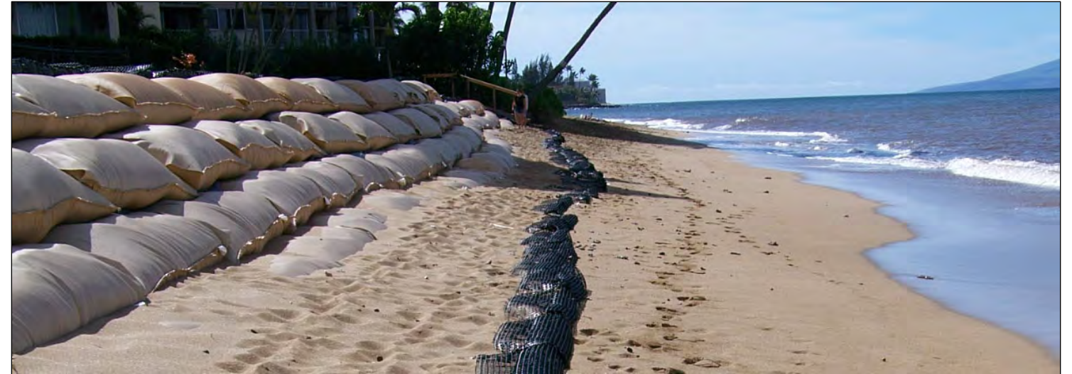
Photo: A sand-filled Elco brand geotextile bag revetment atop Tensor mattresses, West Maui.
