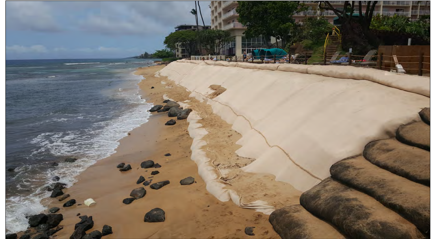
Photo: A geotextile erosion skirt covering an eroded embankment at the Kā’anapali Beach Club, West Maui, 2018.
