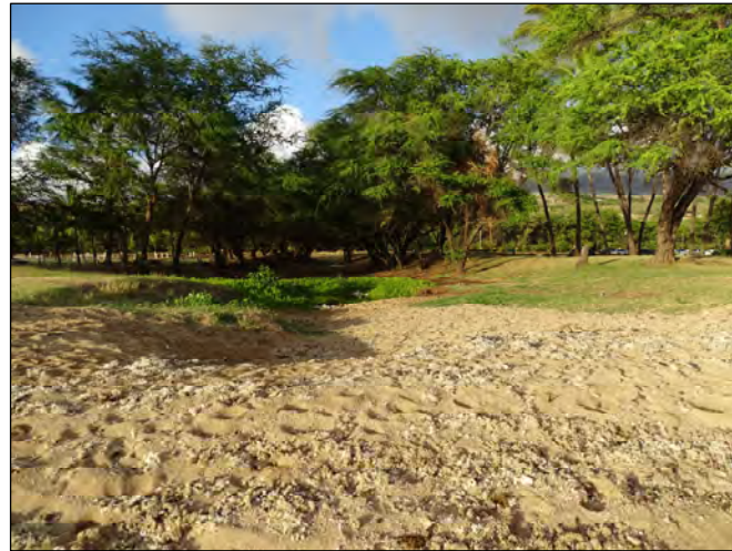
Photo: The sand that plugs this drainage channel could be repurposed for berm enhancement.
