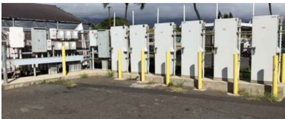
Figure 1. Sunverge SIS BESS + PV units on Maui.
