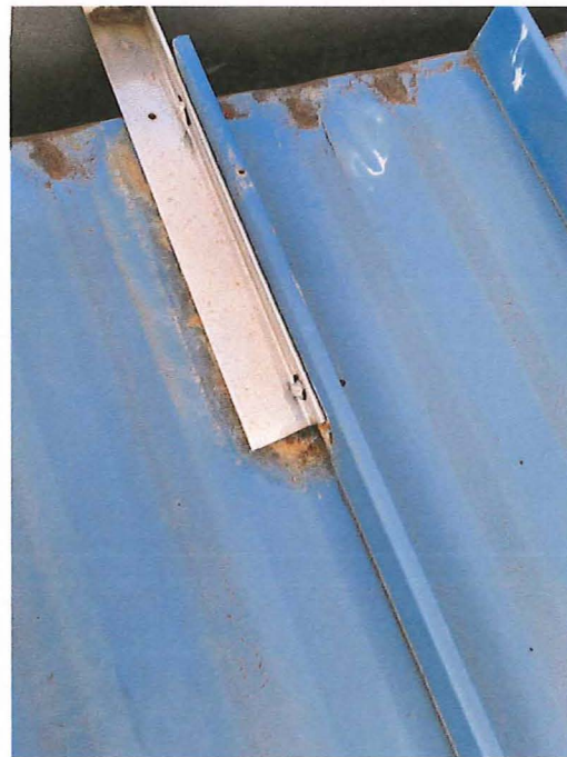
Image 4: Example of gutter bracket rust spot
