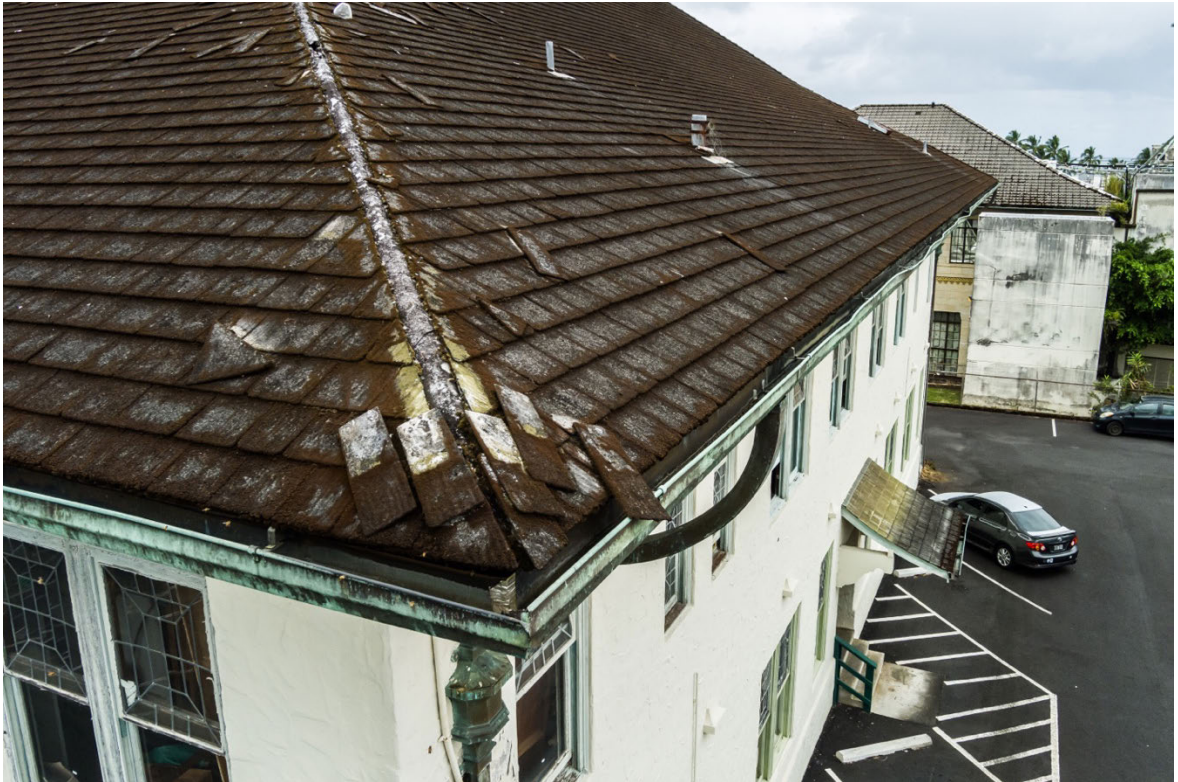
Up close view of the mauka side shingles and dilapated roof. There are bees nested under the gutters on this and the makai side.
