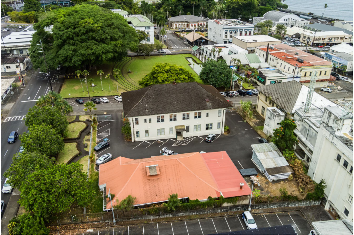
View of the former police station, now East Hawai'i Cultural Center from above. The main building, pictured in the center, has not had roof repair or replacement for over 40 years.
