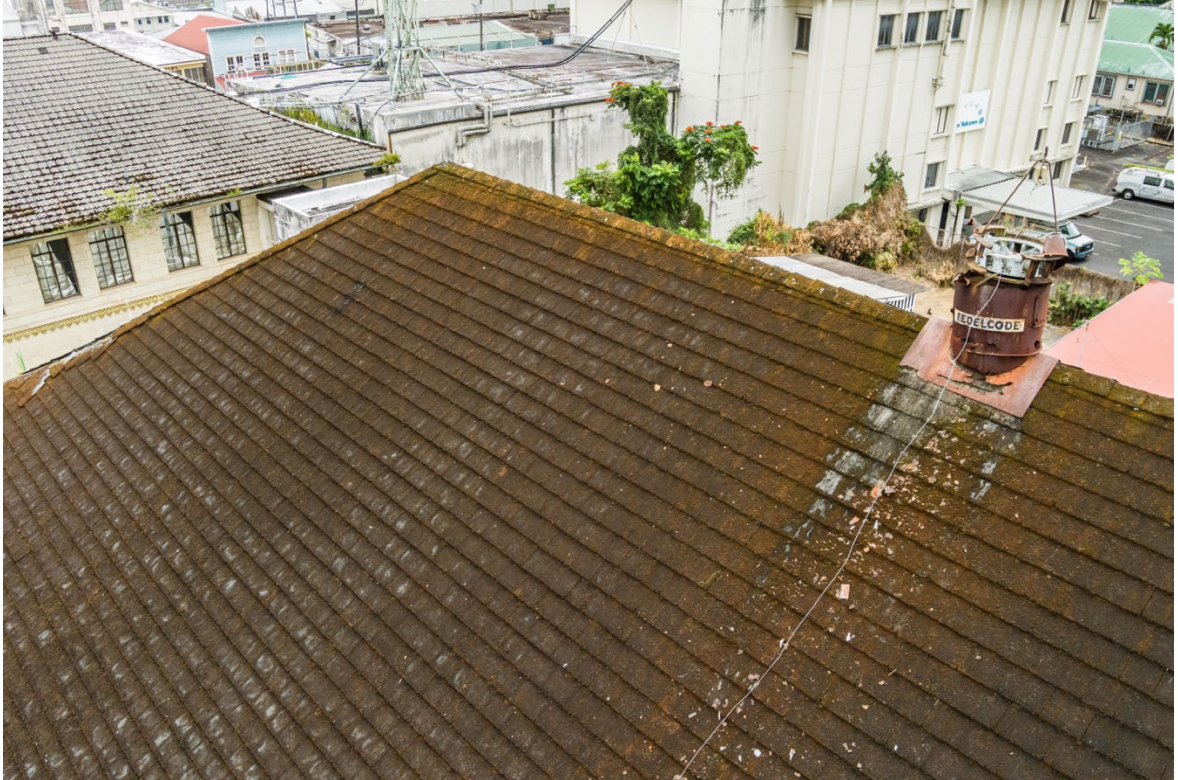
The shingles are sliding and the old temperature control device is rusted and no longer works for effective air flow. The hanging electrical cord is dangerous.
