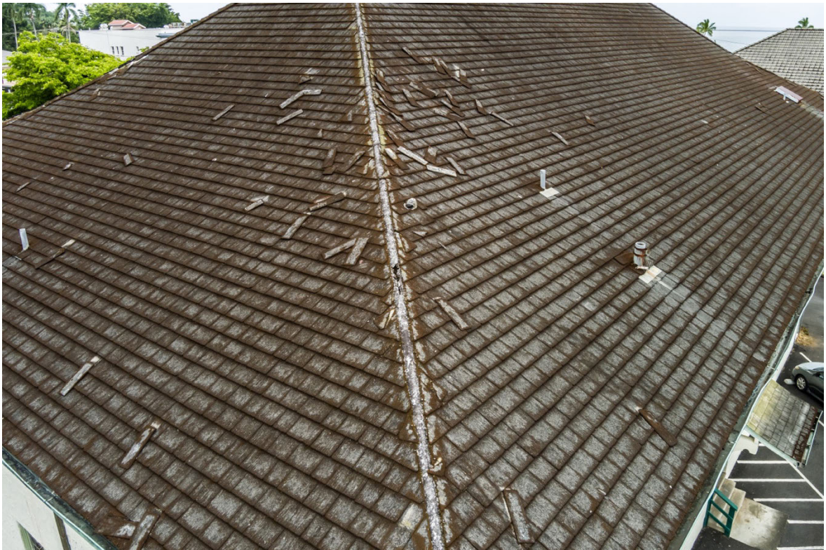
Larger view of the sad state of the roof.
