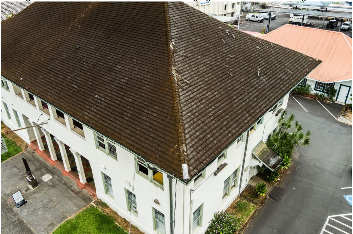
The roof from the front of the building. The seams are cracked and have holes.
