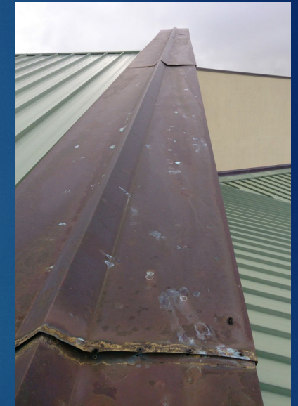
Unsecured and unsealed lap seam in expansion joint.
