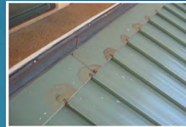
Moderate to severe corrosion of flashing.
