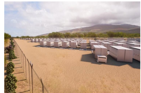
Kapolei BESS Project – DRM site visit January 10, 2023
