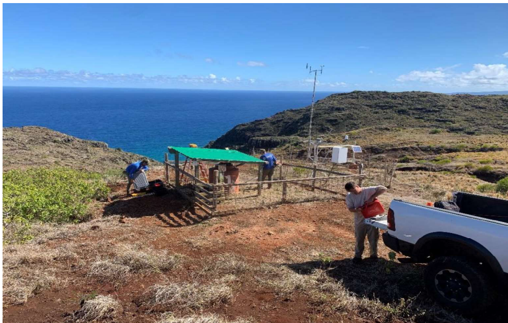
Figure 1. Kuaokala GMA Safety Unit 1 undergoing repairs for gutter system, paint, and vegetation management.
