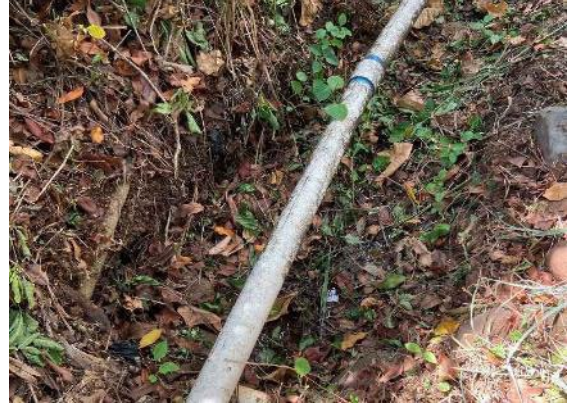
B) An old section of a County water line sits in the ‘auwai, where the water stops flowing approximately 900 feet before the first kuleana user.
