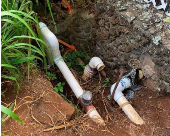
A) Distribution pipe with valve chained and flow meter at center, located on the boundary of Imua Family Services property.
