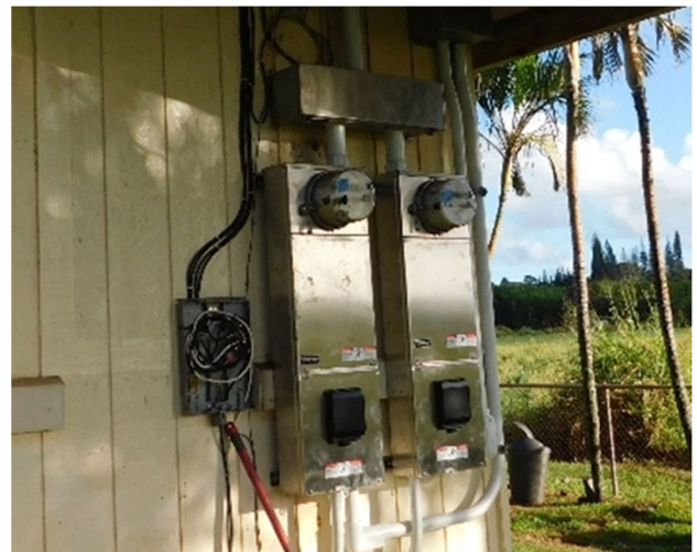
New electrical boxes
