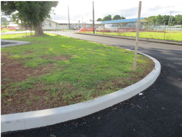
Parking lot without security/safety lighting
