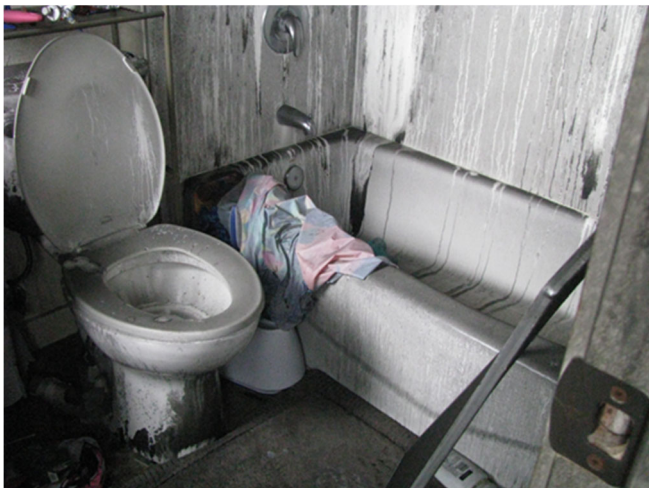
Smoke damaged, 2nd floor bathroom
