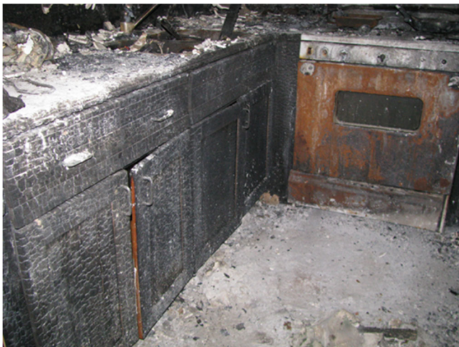
Damaged kitchen, source of fire
