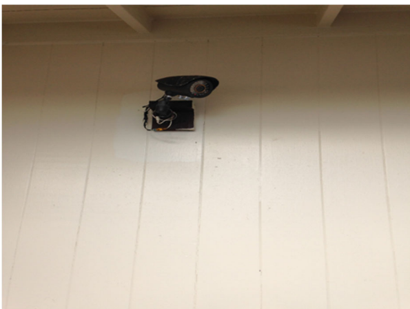
Old security system at AMP 37 office
