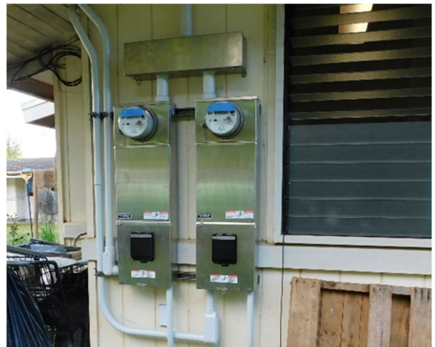
New electrical boxes
