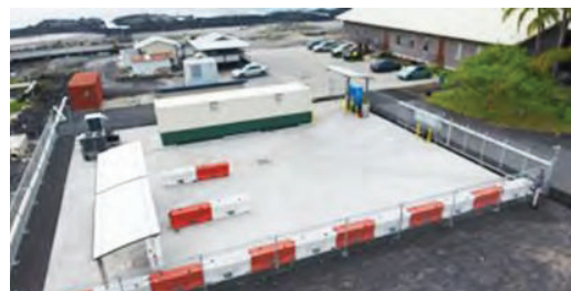
Figure 3. HNEI Hydrogen Station.
