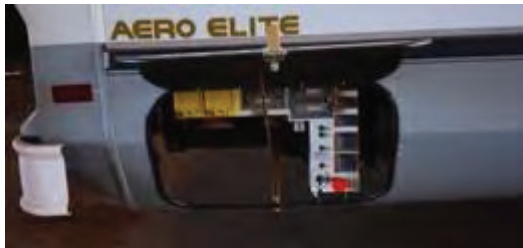
Figure 9. Bus Export Power Unit.
