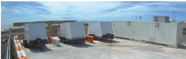
Figure 5. Hydrogen Transport Trailers.
