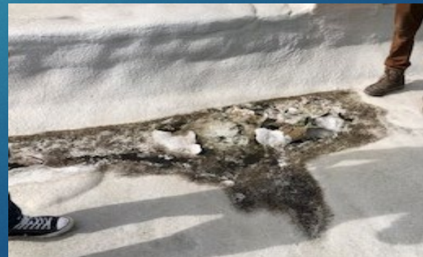
Exposed blisters with deteriorated coating and foam
