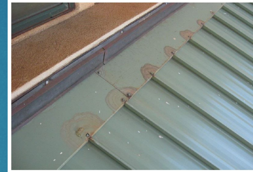
Moderate to severe corrosion of flashing.
