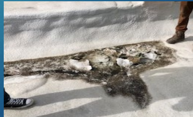
Exposed blisters with deteriorated coating and foam
