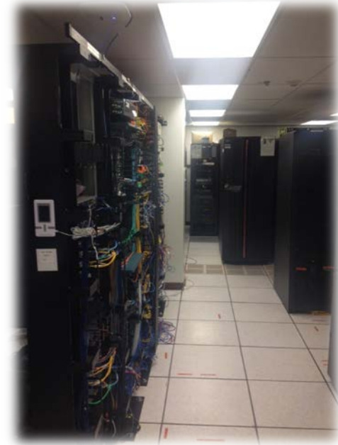
(Right) Data Center
