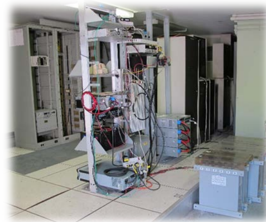
(Below) Communication Racks
