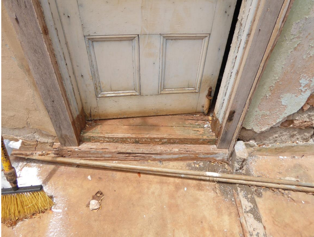
Figure 34: Sill of Door "E". Note remnant of concrete curb and deteriorated plaster which exposed coralline wall construction.
