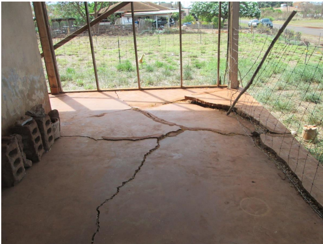
Figure 49: Damage to deck at southeast corner. Photo taken in 2015.
