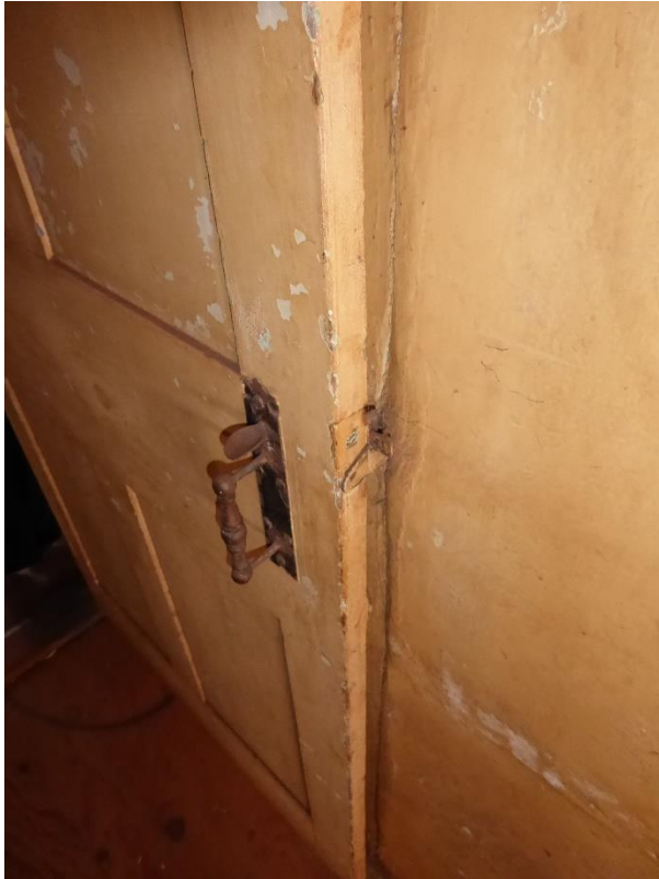
Figure 35: Holdback hardware at door L.
