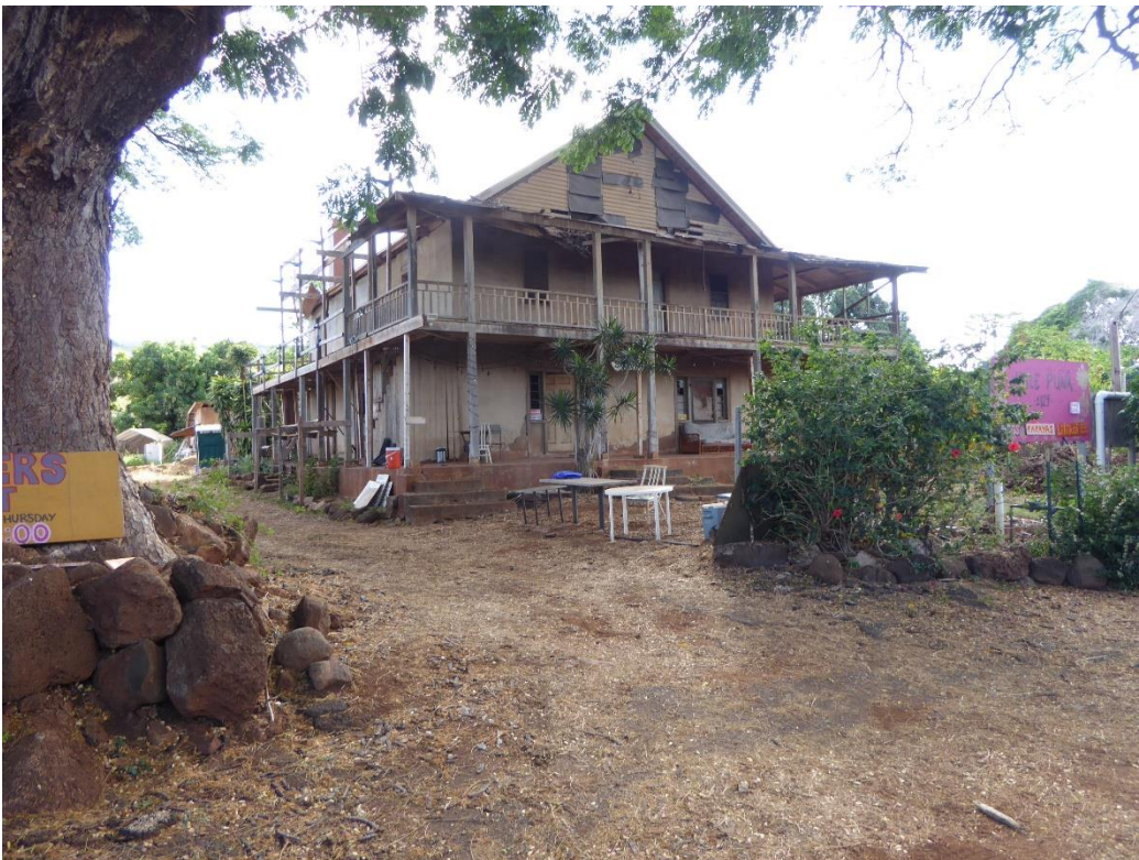
Figure 11: Photo taken in 2019. Note gable roof eave and missing roof over west deck.
