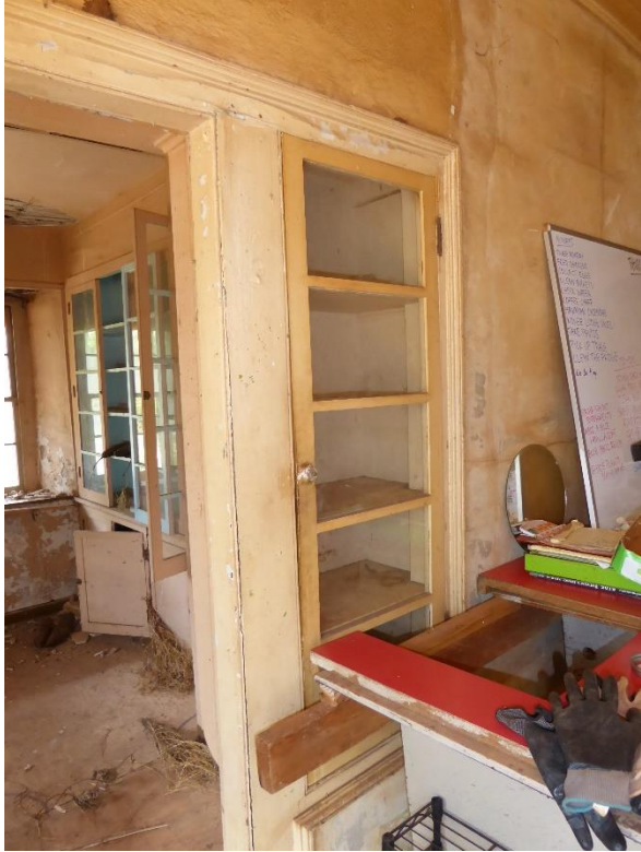
Figure 42: One of the two cabinets in the Dining Room flanking Door G. This cabinet has a door. The other cabinet is missing its door.
