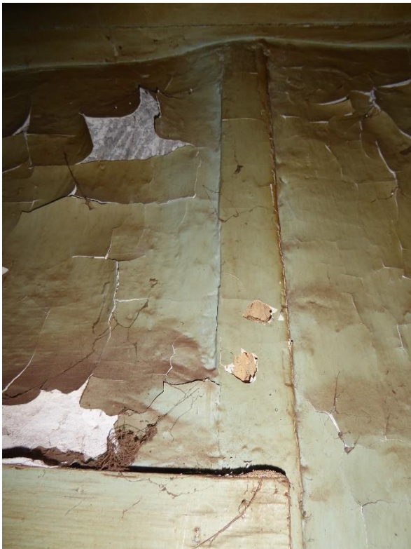
Figure 17: Original stud shows on interior of Kitchen, with shallow scalloped plaster wall between studs.
