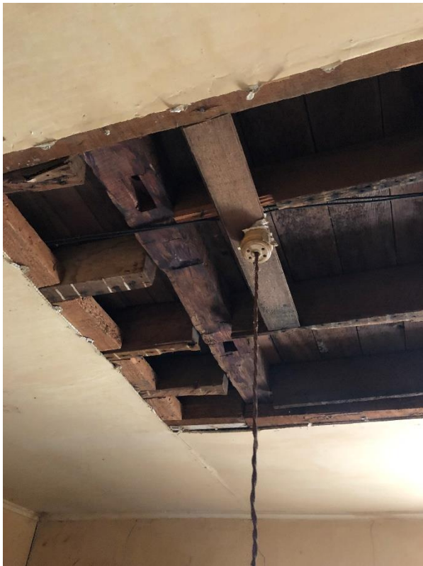
Figure 7: Ceiling in bathroom is 14" thick gypsum board attached to original hand-hewn framing.
