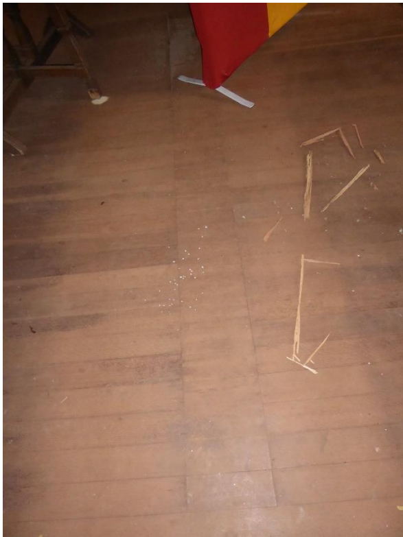
Figure 21: Patch in the floor of the Parlor where the wall was removed.
