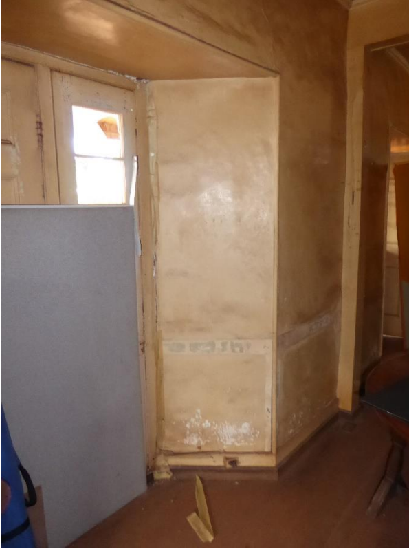
Figure 16: Shadow of former wainscot trip is evident on this portion of the east section of the Parlor.
