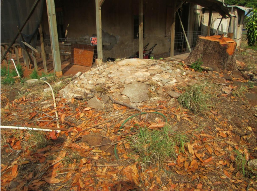
Figure 9: Cistern. Photo taken in 2015, prior to collapse of north shed roof structure.
