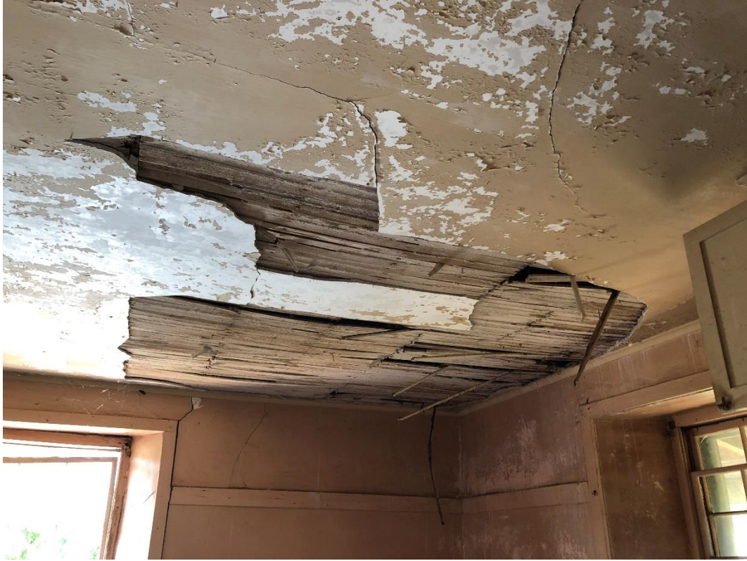
Figure 24: Typical ceiling damage at second floor.
