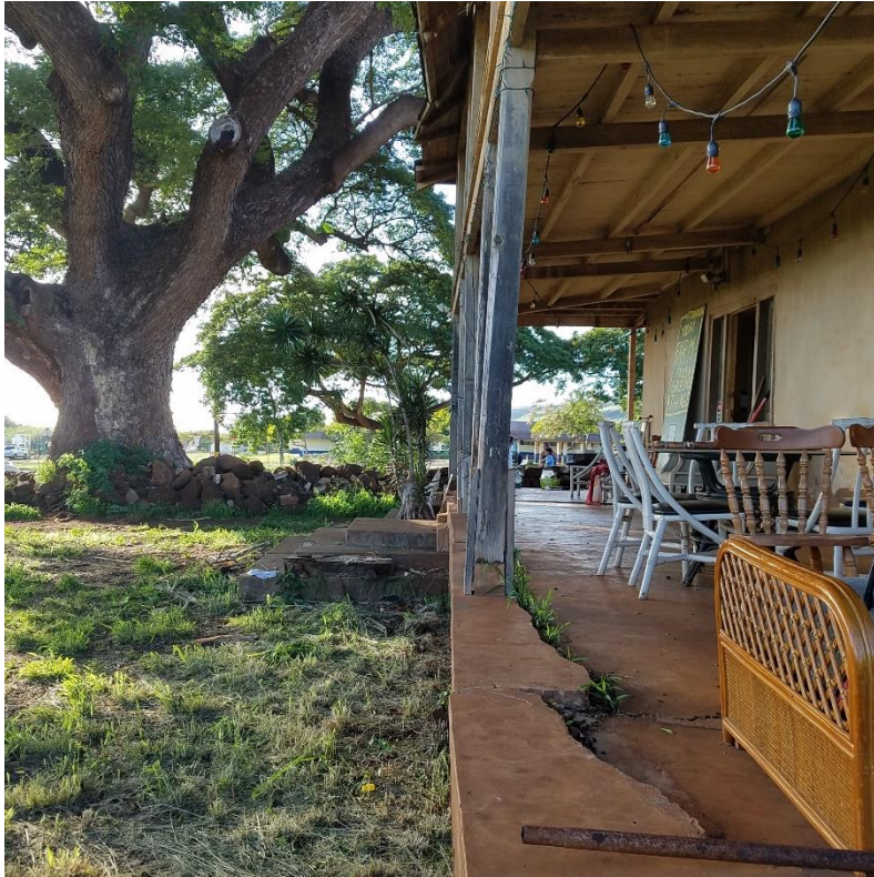
Figure 50: Retaining wall separating from deck and leaning south. (Taken 2015)
