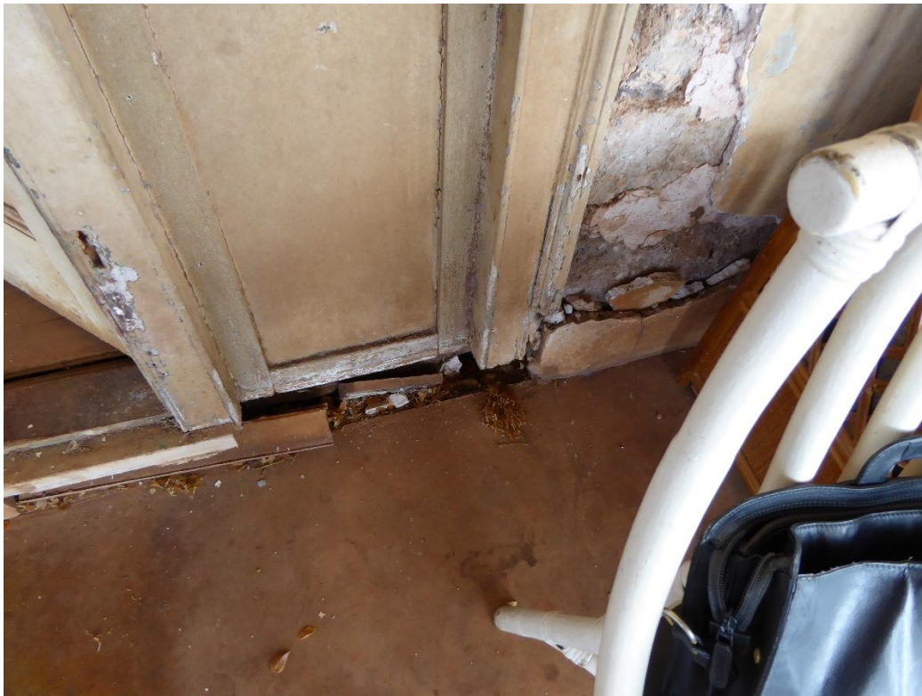
Figure 13: Plaster adjacent to south door has failed. Note cement plaster remains at base.
