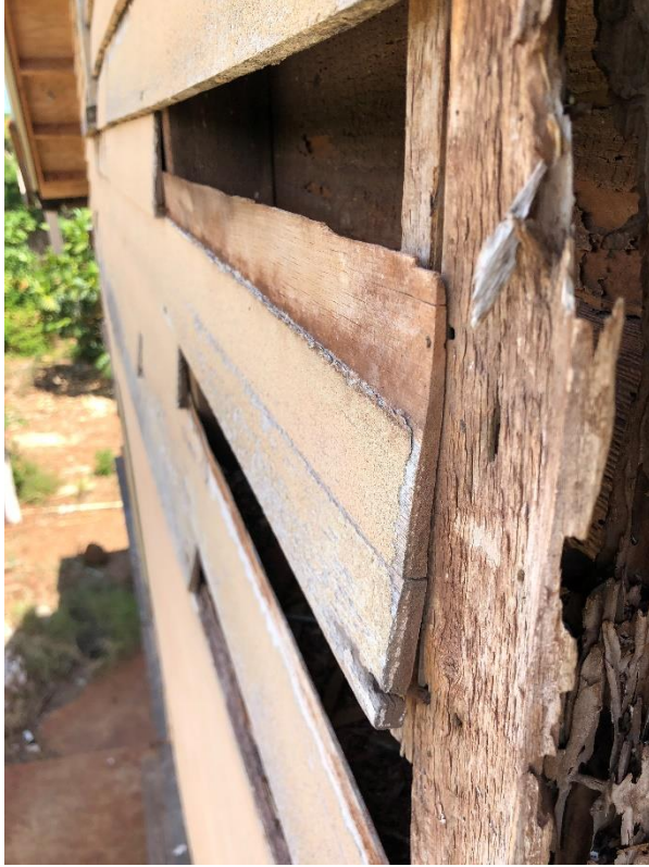
Figure 12: Siding on north gable wall near window
