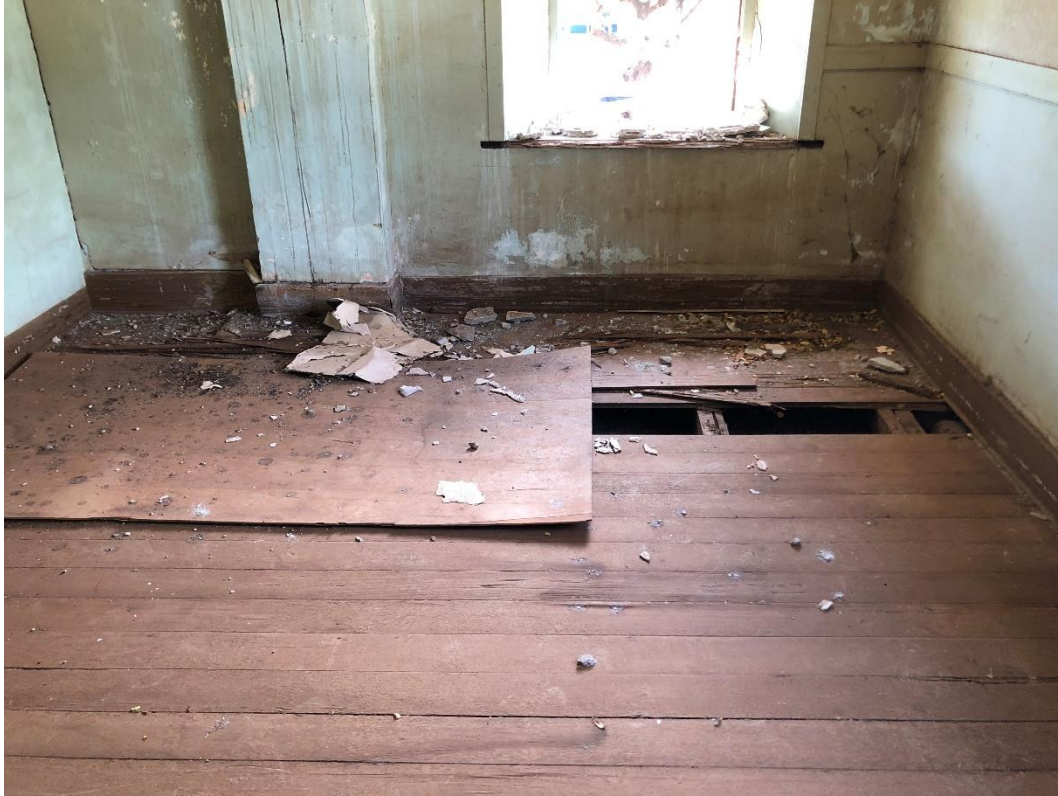
Figure 22: Damaged floor in bedroom 3. Note the wall thickness change at the chimney
