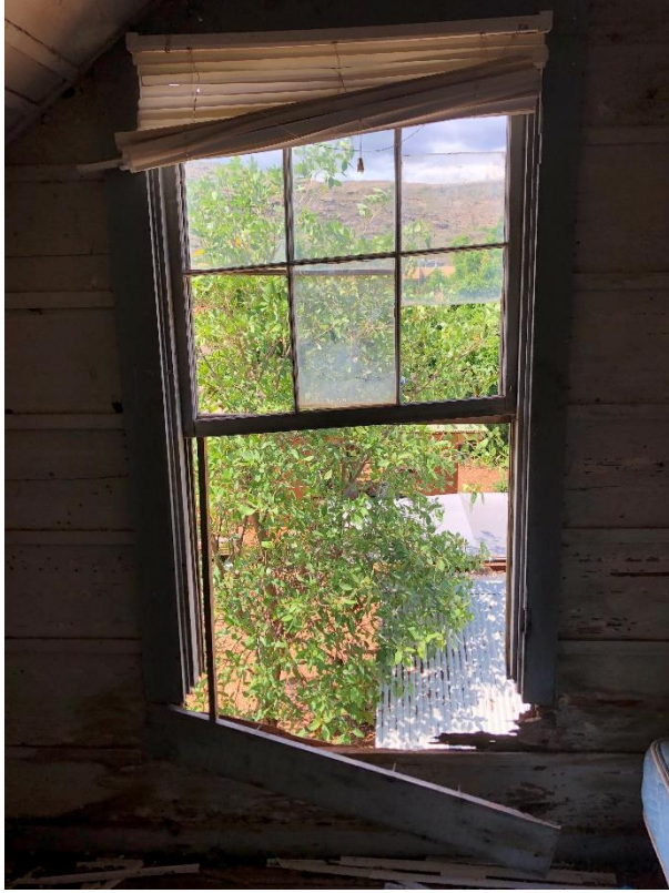
Figure 30: Window 31 sash is close to collapse.
