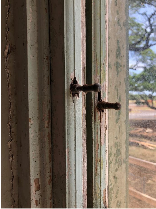
Figure 26: Window 28 is the only window with this type of spring sash holder.
