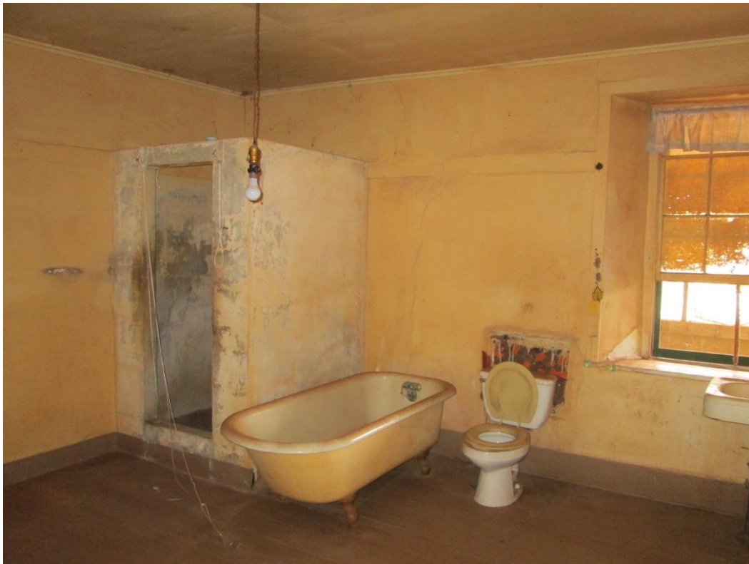
Figure 53: Bathroom showing toilet, tub, and shower. Part of sink is shown on the right.
