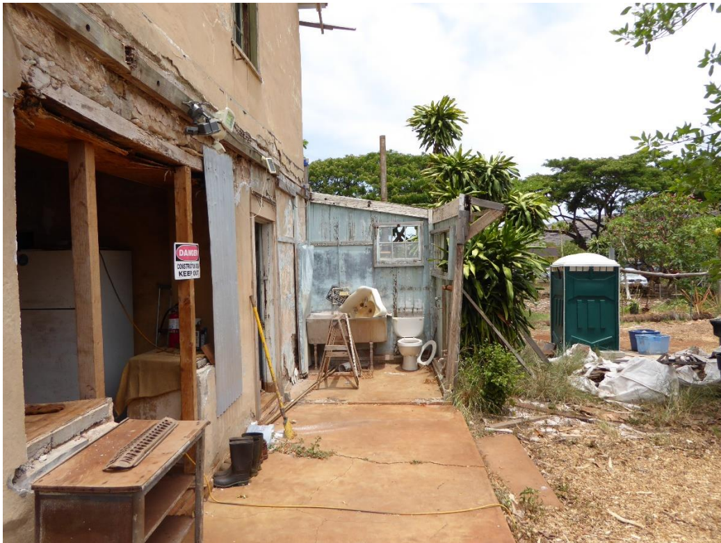
Figure 15: Lintel over opening at left on north side. Remains of the washroom beyond.
