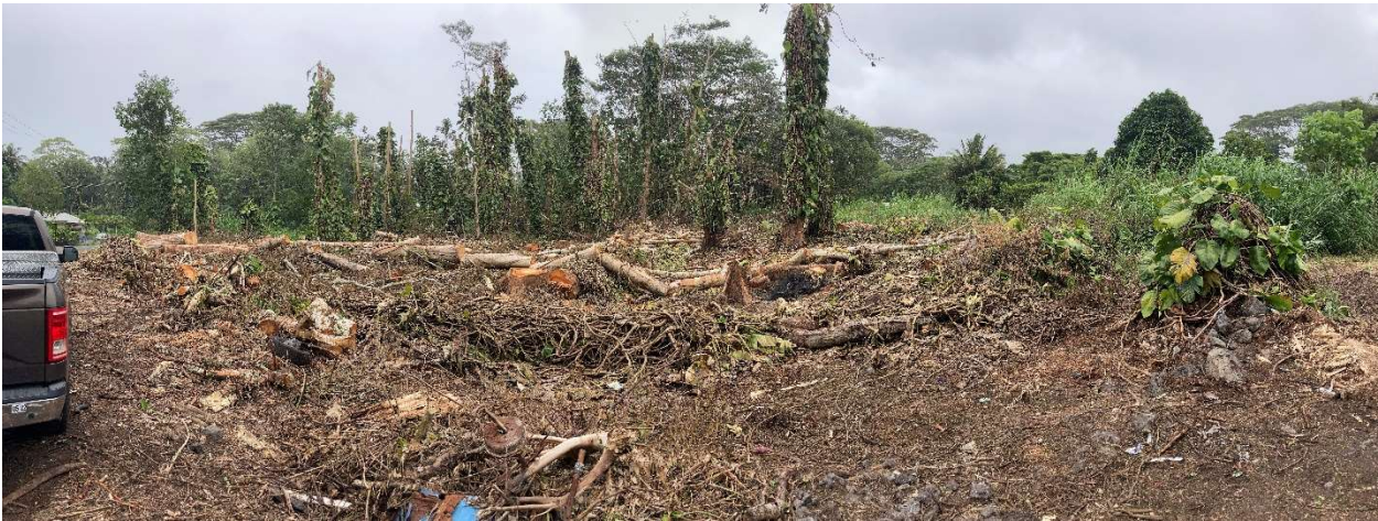
Photos of Site 12 & 13 after removal, from the opposite end of the road. Staff are circled in yellow.
