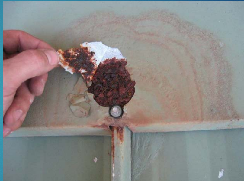
Blistering coating, corrosion of underlying ferrous metal
