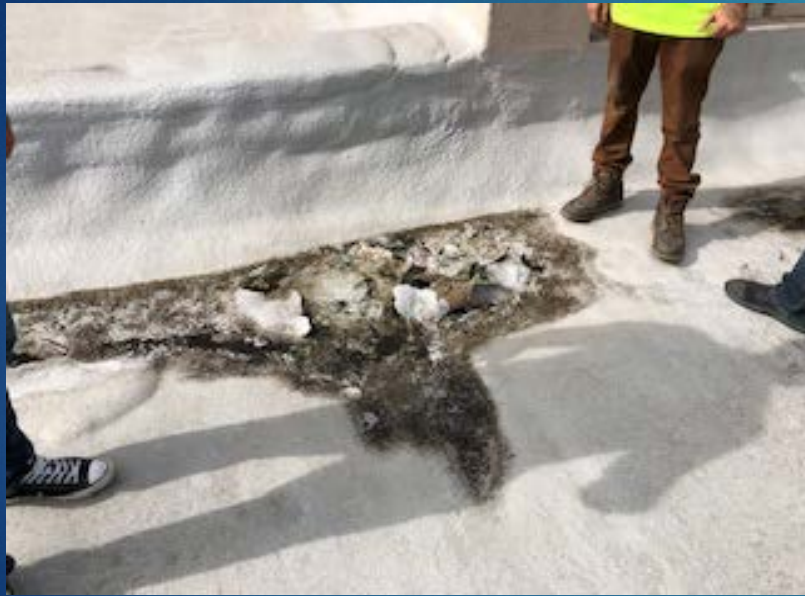
Exposed blisters with deteriorated coating and foam
