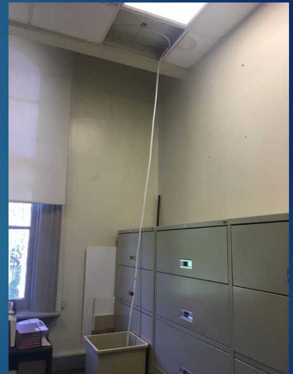
Temporary catchment with water draining into trash receptacle
