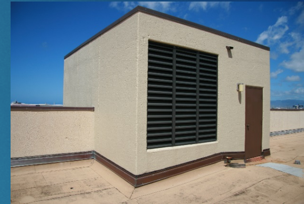
Machine room air cooled through wall vents
