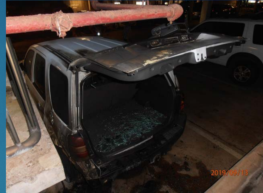
Burnt State vehicle under failed sprinkler head
