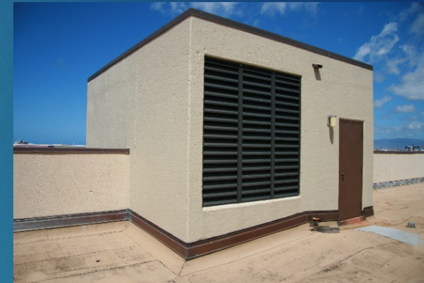
Machine room air cooled through wall vents
