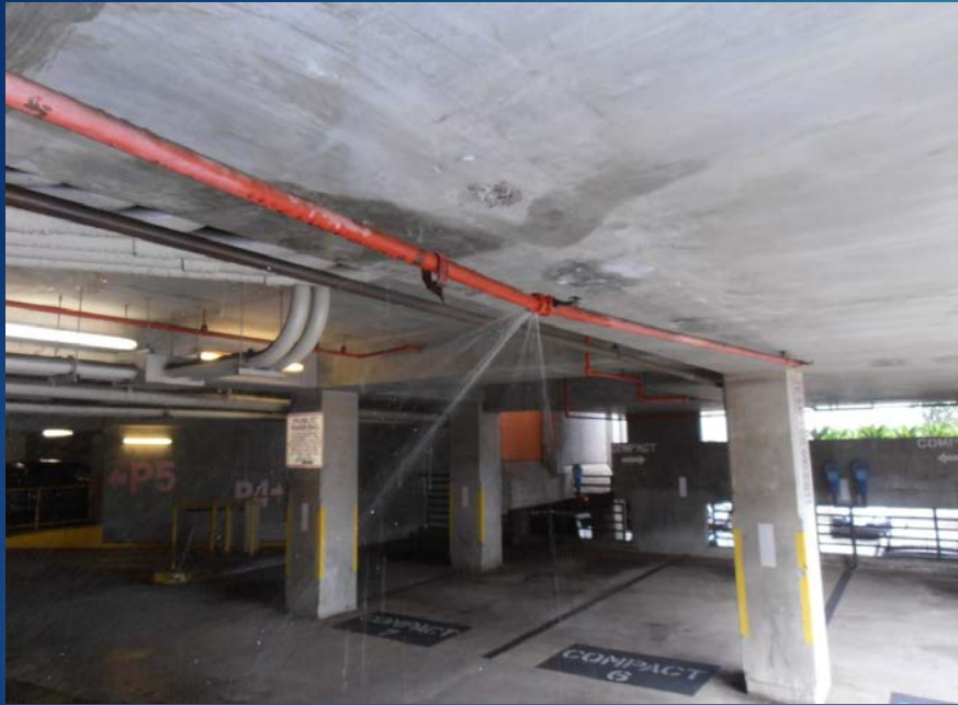
Failed sprinkler system joint Note: Hanger support has corroded and failed
