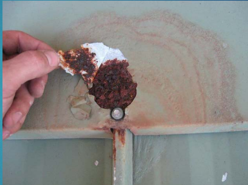
Blistering coating, corrosion of underlying ferrous metal
