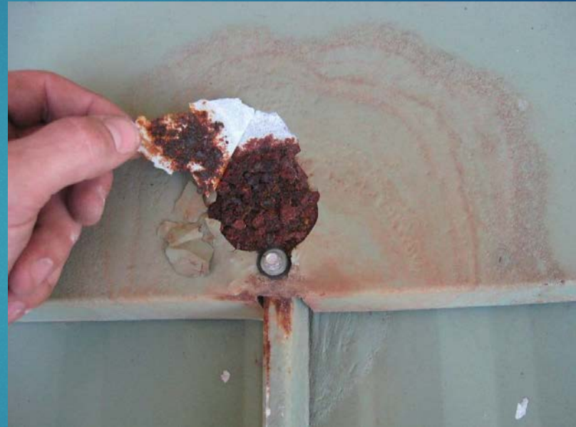
Blistering coating, corrosion of underlying ferrous metal
