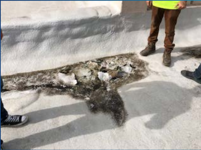
Exposed blisters with deteriorated coating and foam
