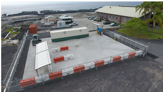
Figure 1. NELHA 65 kg/day Hydrogen Station
