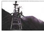
1958 The first 138 kV lines are strung from Waiau over the Ko'olau range. The Pali tunnels and a new highway open Windward O'ahu to development.
