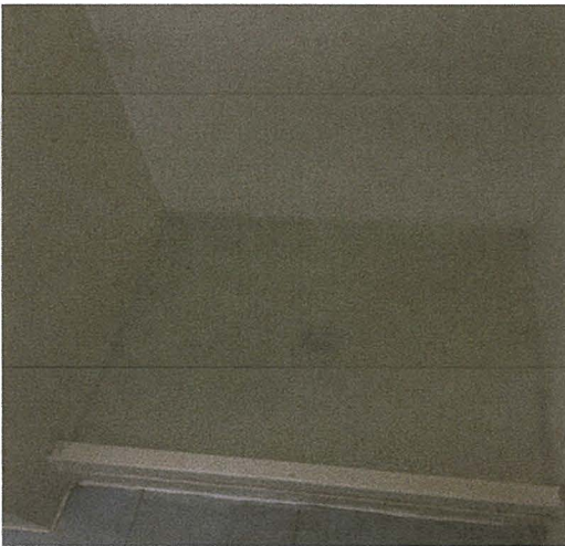
3. Clog Shower Drain located on the 2 nd floor unit
