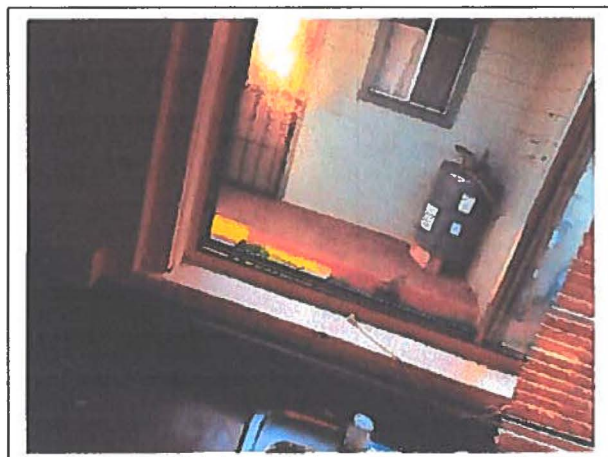
New water heater & other major appliances
