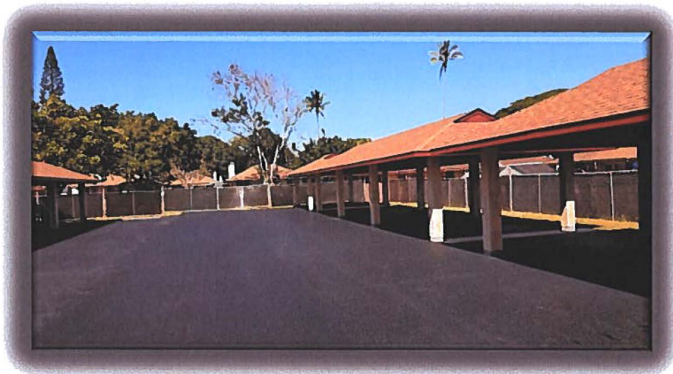
Wheeler Army Airfield – Island Palms Community Scope: Asphalt Mill and Repave and Stripe Contact: Lendlease
