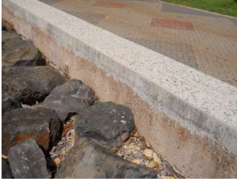
SHORELINE REVETMENT ALLOWS SAFE PUBLIC LATERAL ACCESS
