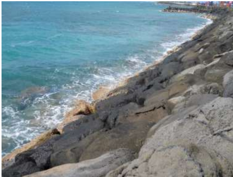
SHORELINE REVETMENT PREVENTS SAFE PUBLIC LATERAL AND OCEAN ACCESS
