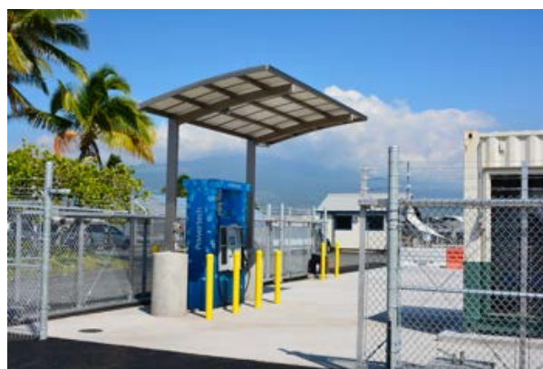
Figure 4: NELHA Hydrogen Station Dispenser
