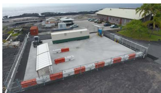
Figure 2: NELHA Hydrogen Station Aerial View
