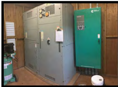
▲ New Automatic Transfer Switch (ATS) for the Honokahua B site
