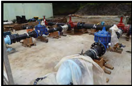
▲ Upper Kimo pumps
