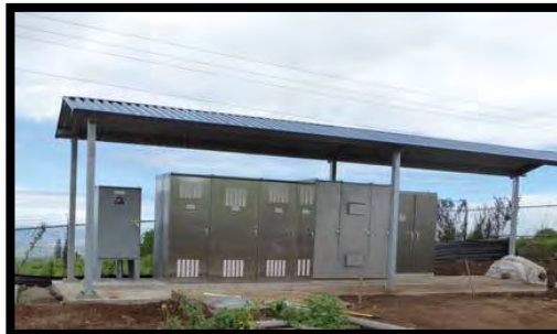
▲ Middle Kimo electrical equipment
