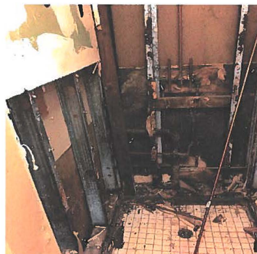
Water Damage Shower Area
