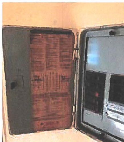
New Wiring & Circuit Boxes in some units
