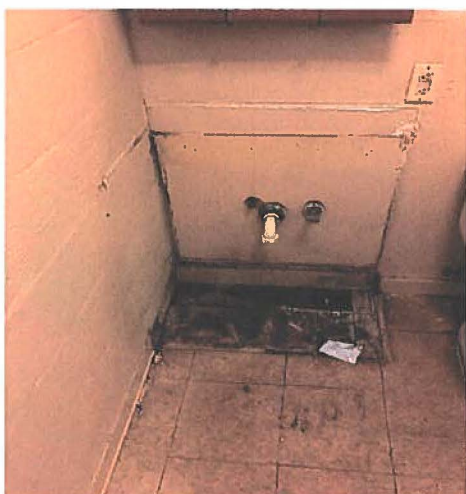
Bathroom Floor Damage
