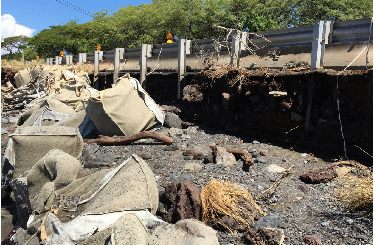
At left center of this photo, the guardrail supports are hanging in the air. Erosion has undermined the pavement by several feet in some places. Temporary erosion control bags have been scattered by wave action.
