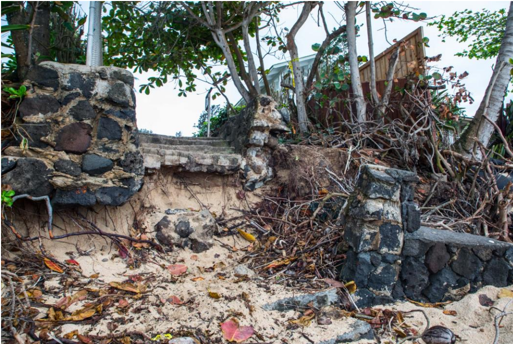
Figure 3: Eroded and destroyed beach access points on North Shore O'ahu
