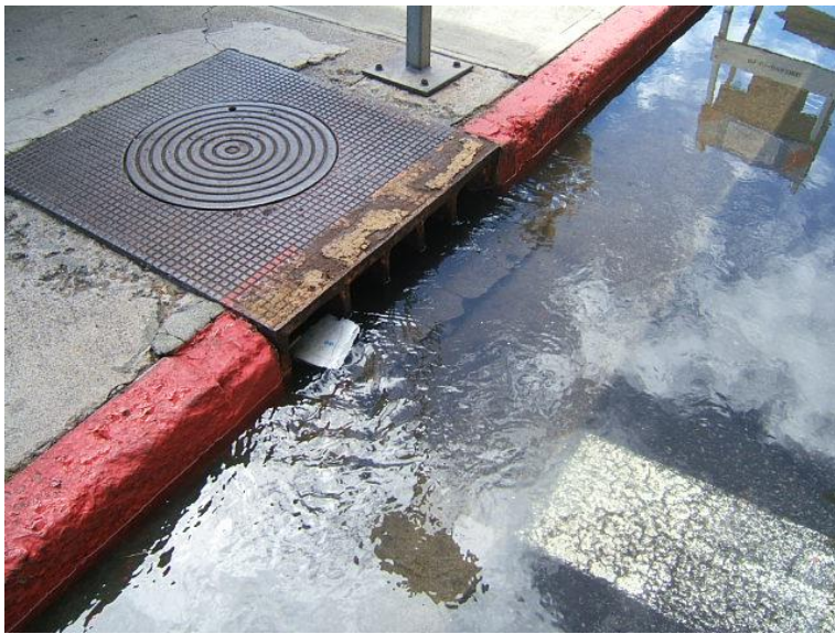
Street drain seawater backflow
