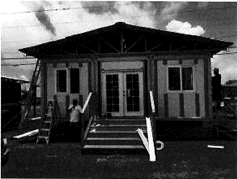
Trusses and roofing is installed and walls are framed out ready for exterior paneling.
