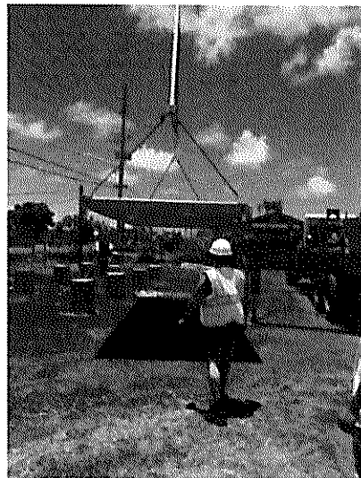
Using a winch crane to set the 2000 lb concrete board floating on the foundation.
