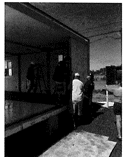
Installing the (optional) Insulated Panels (IP) to create the (optional) second story.
