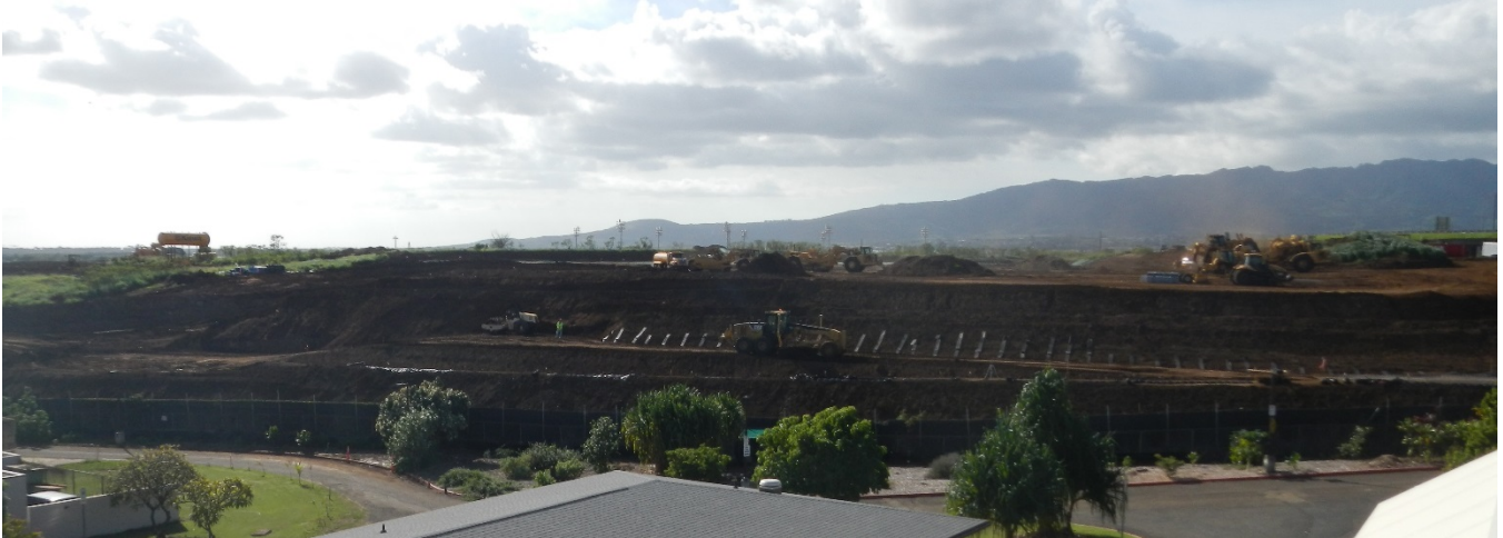
Amazing Transition – Rail Operations Center at the Former Ewa Junction Fuel Drumming Facility under Construction in 2013
