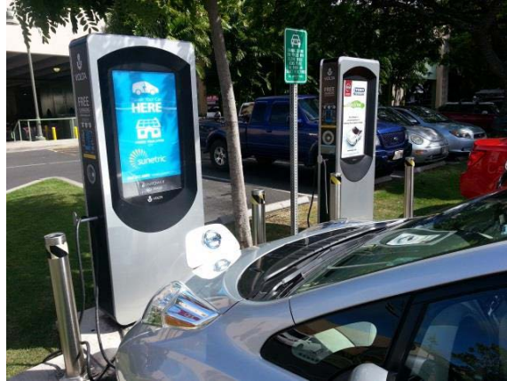
Figure 7. EV charging stations in Kailua, O'ahu.
