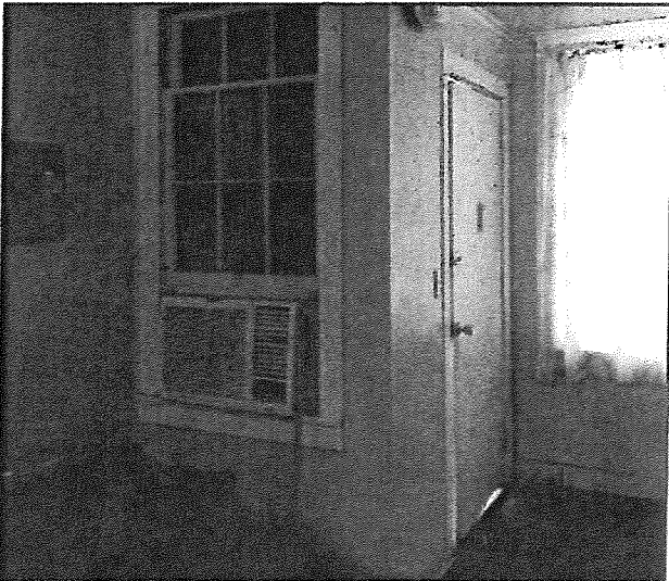
Figure 27. Door frame not square
