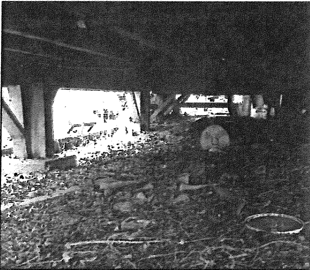
Figure 2. Severely damaged floor girder
