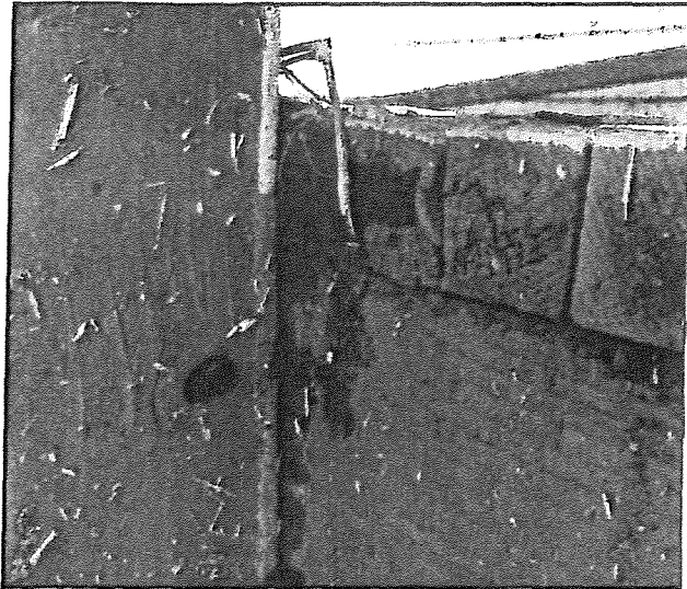
Figure 6. Damaged ramp floor boards
