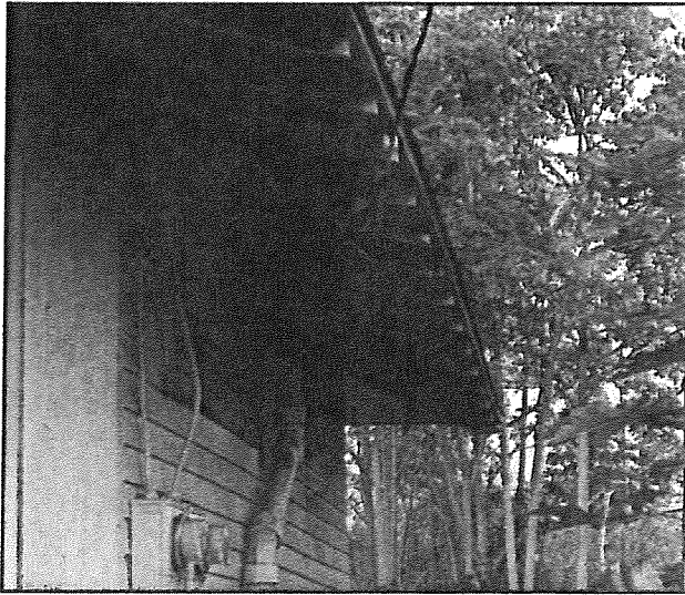
Figure 14. Damaged rafters; uneven roof lines
