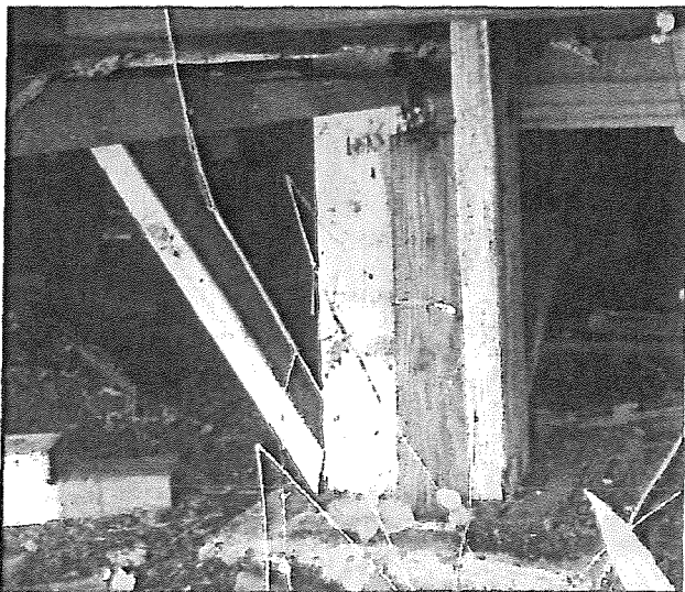
Figure 10. Damaged structural members
