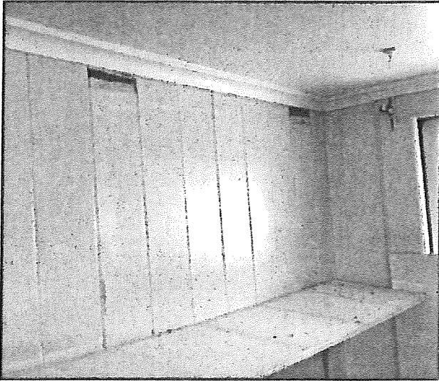
Figure 29. Unattached wall boards (structural)
