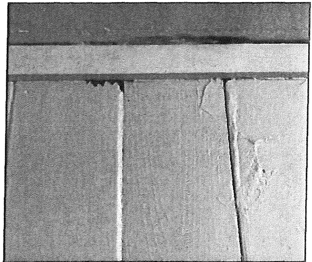
Figure 21. Possible water damage
