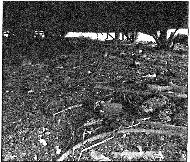
Figure 3. Sagging floor girder (in background)
