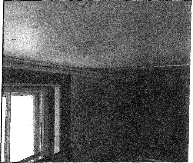
Figure 19. Possible water damage
