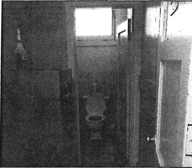
Figure 25. Non ADA compliant bathroom
