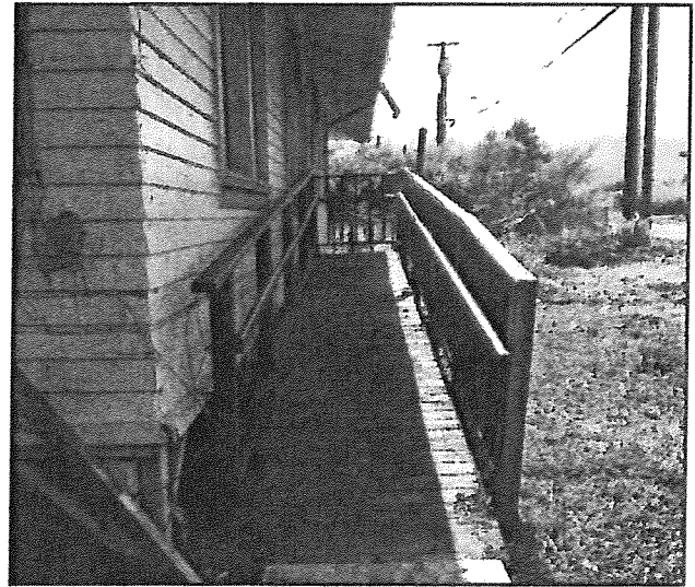
Figure 15. Unusable access ramp
