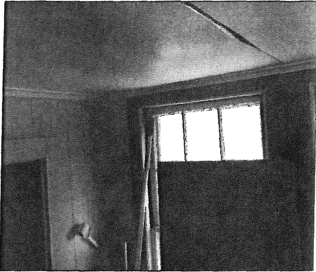
Figure 18. Possible water damage
