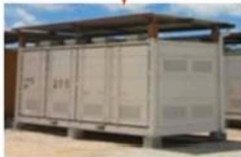
PPES Battery Storage (BESS)
