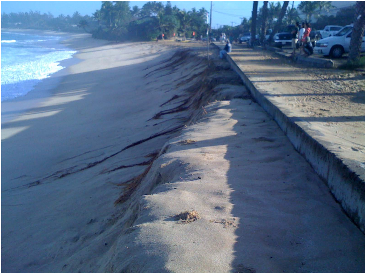
Erosion at Sunset Beach Bike Path
