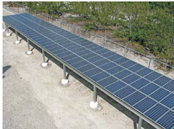
FKEC's Marathon Array (left) and Crawl Key Array (above). Photos courtesy of FKEC.
