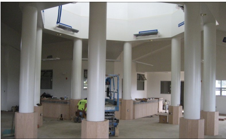
Workers put finishing touches on the construction of the new Kohala Library.
