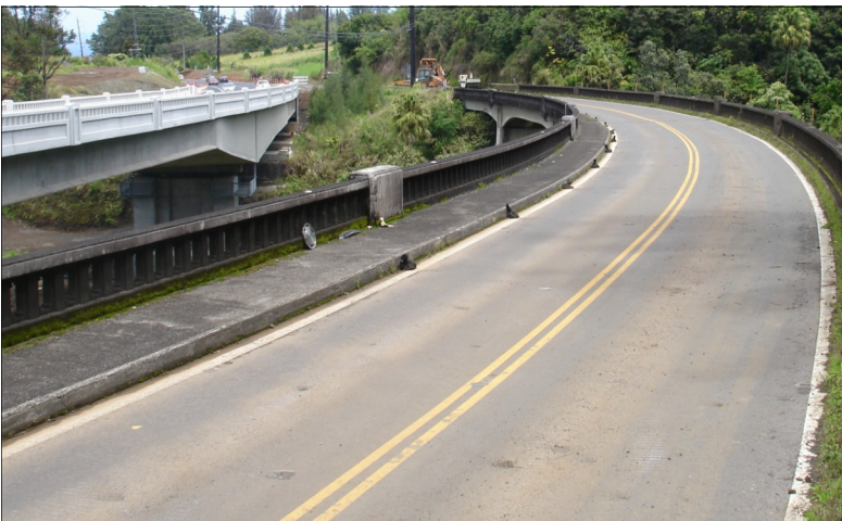
The old Kealakaha Bridge stands silently after years of service as two way traffic flows over the newly opened Kealakaha Bridge.
