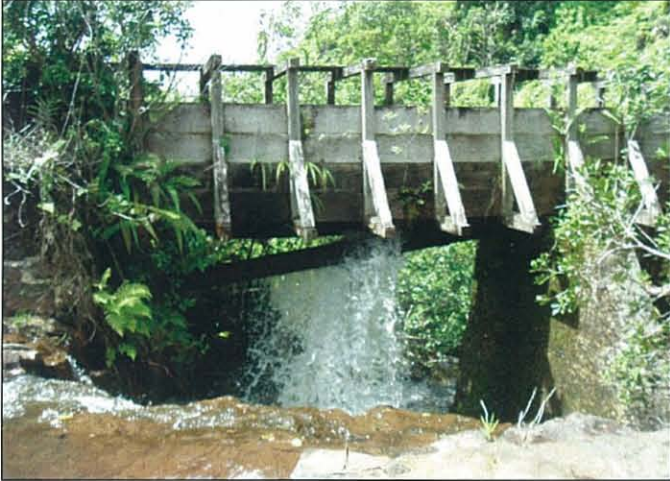
This main transmission line flume suffered serious damage during a flood
