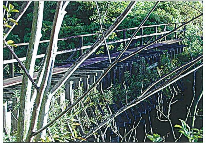
This deteriorated 80-foot redwood flume carrying water from Wailua Reservoir to Kapaa over the deep Opaekaa stream ravine was replaced in a CIP project with a pipe.
