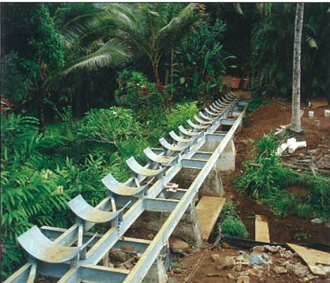
Steel supports installed for a piped replacement of a redwood flume at Kapaa stream
