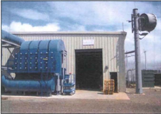
Xtreme Power BESS Building Entrance (Looking SE)
