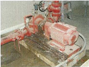
Deteriorated Existing Fire Sprinkler Pump
