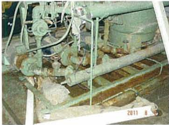
Deteriorated Existing Domestic Water Booster System Equipment
