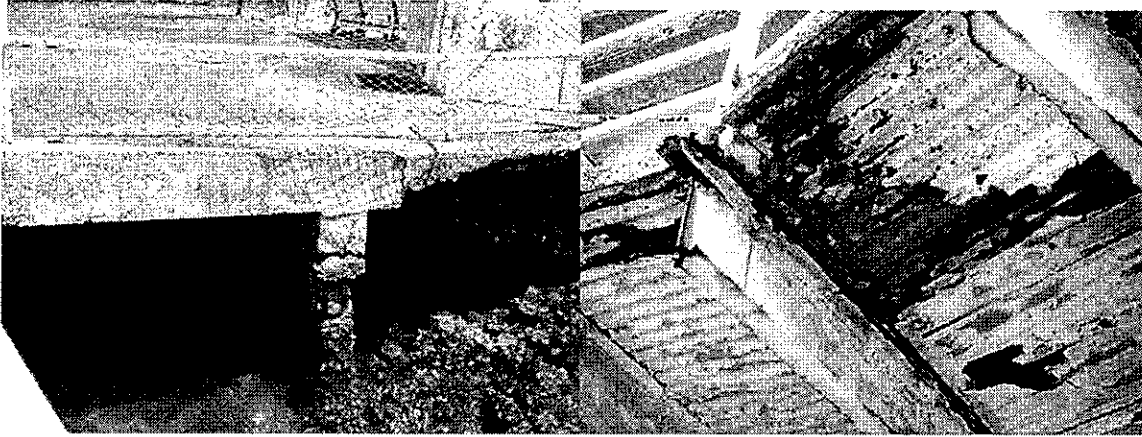
Pier support columns are eroded,unsafe Walkways on buildings are rusting, unsafe.
