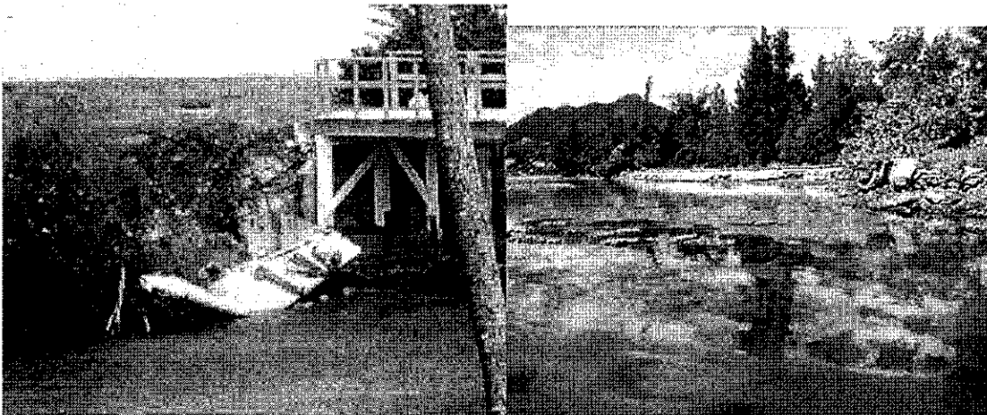
Fallen seawall, inner lagoon
